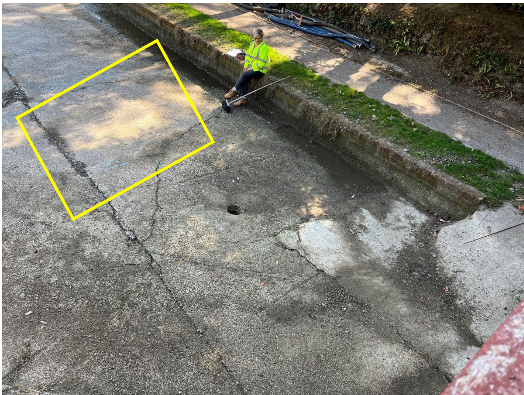
Plate 2 – View to upstream end of pond showing voided area A12.
