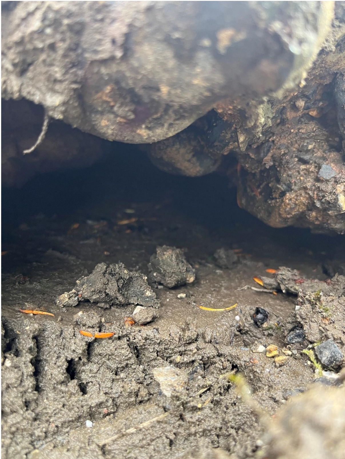
Plate 9 – Wash out and voidage at sinkage area to area A4.
