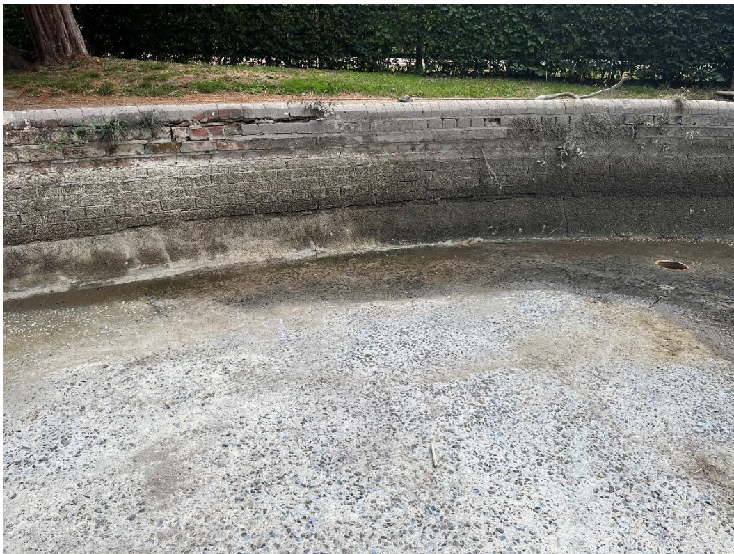
Plate 6 – Voided area to slab at area A9, adjacent to pond wall.
