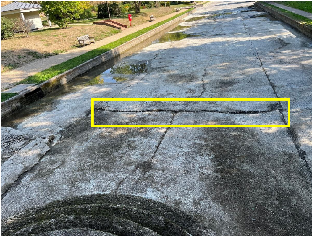
Plate 1 – View from upstream end of pond showing cracking and voided area A15.
