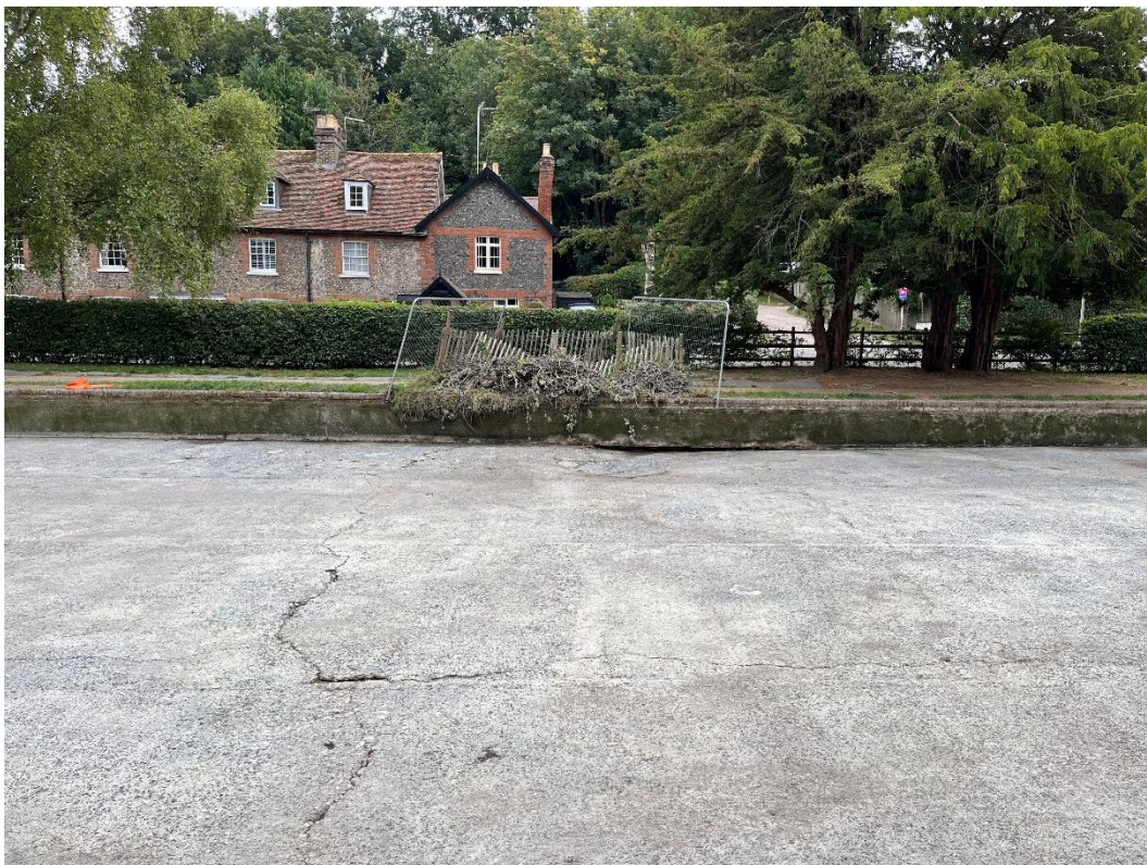
Plate 8 – General view to sinkage and voidage at area A4.
