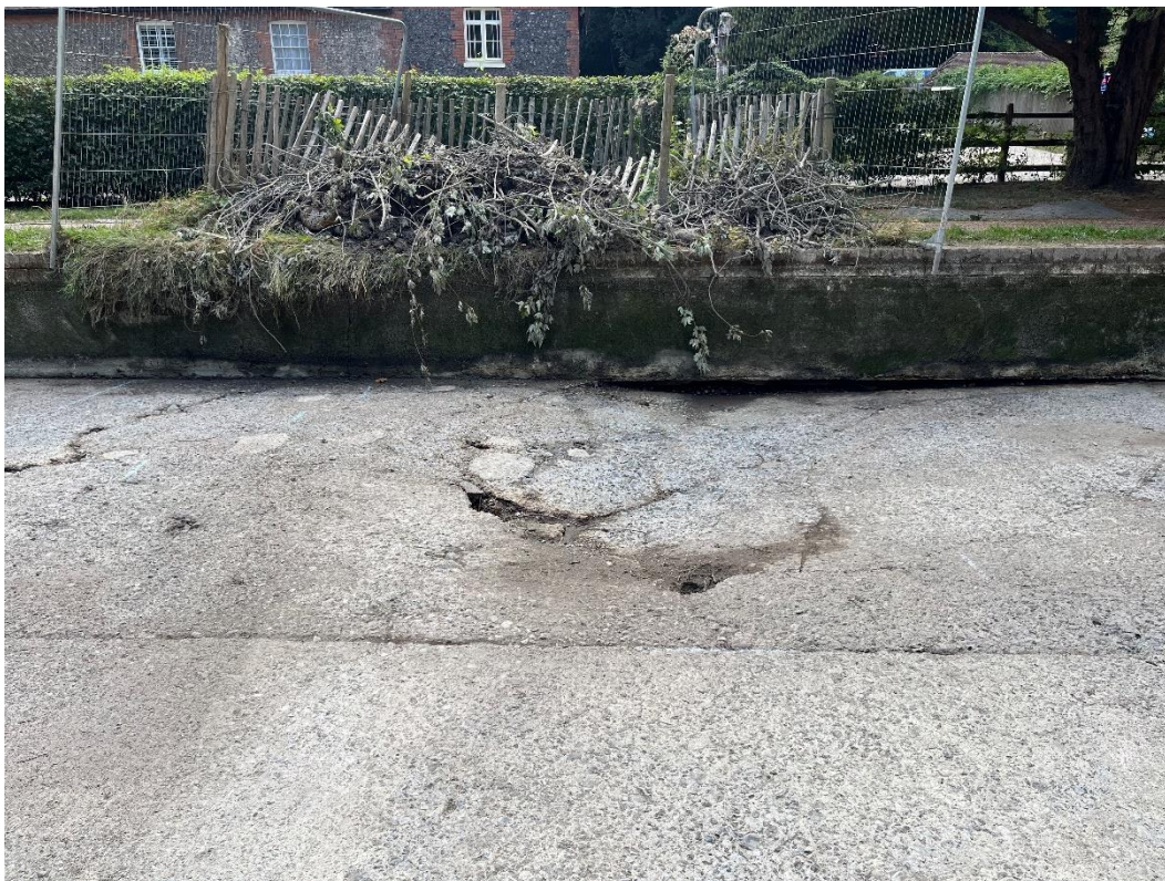
Plate 4 – Showing voided area and failed slab to area A4.
