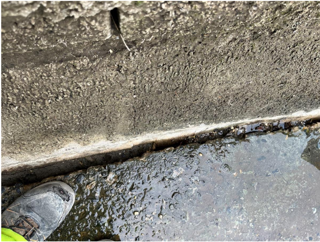
Plate 7 – Voidage at wall / slab interface at area A9.
