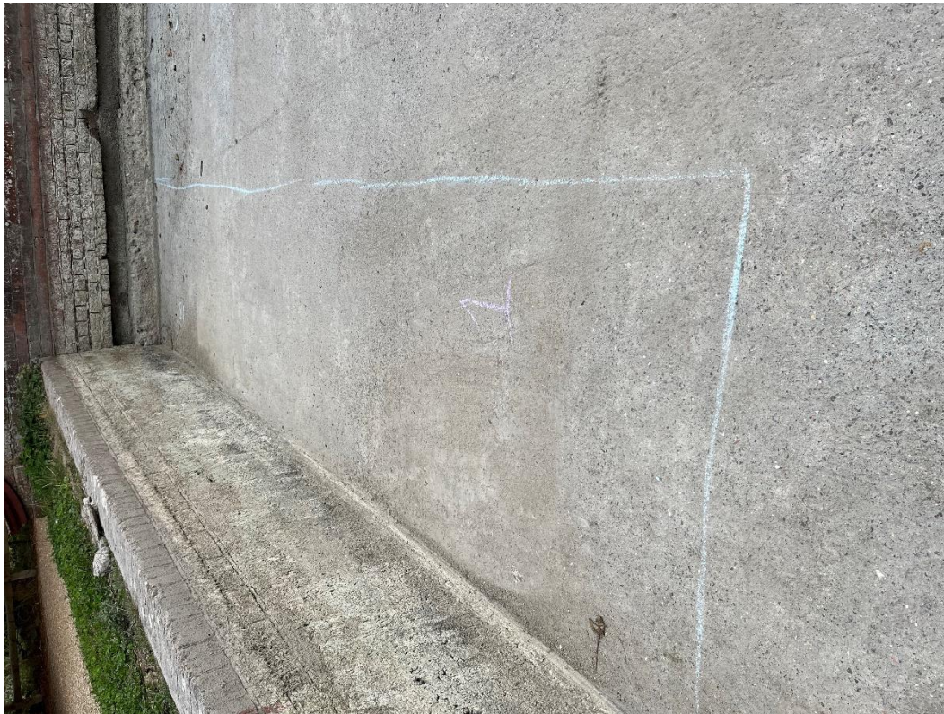
Plate 3 – Showing voided area to downstream end of pond at area A1.
