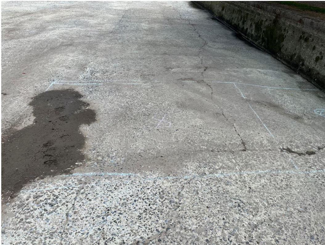
Plate 5 – Voided area to slab at area A8.
